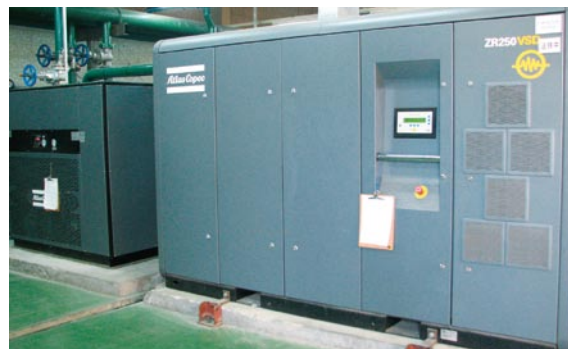
Photo 6: Compressor at Kunshan NSK
