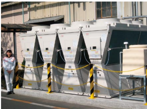
Photo 2: High-efficiency heat pump chiller unit installed through the efforts of the Air-Conditioning Systems Working Group
