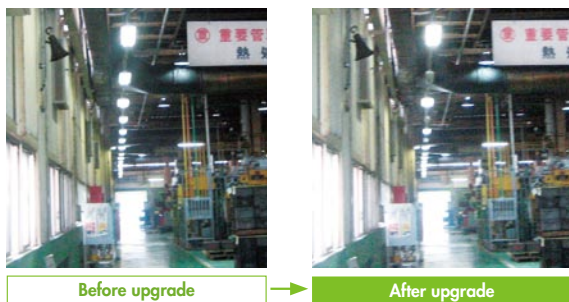
Photo 5: Thinned out ceiling area lighting
